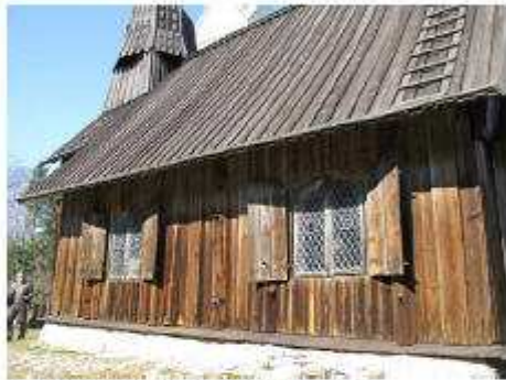
Fig. 8. Exterior panelling with HB attack
