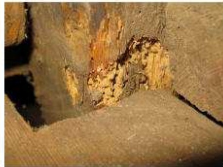
Fig. 5. Detail of altar (interior, XR damage)
