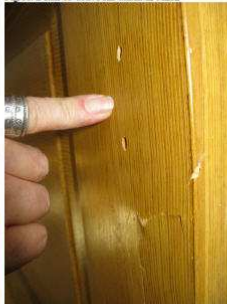
Fig.13. Emergence holes and loose surface layer
