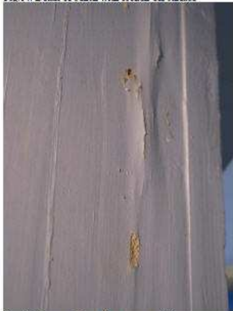
Fig.16. Loose surface with emergence holes
