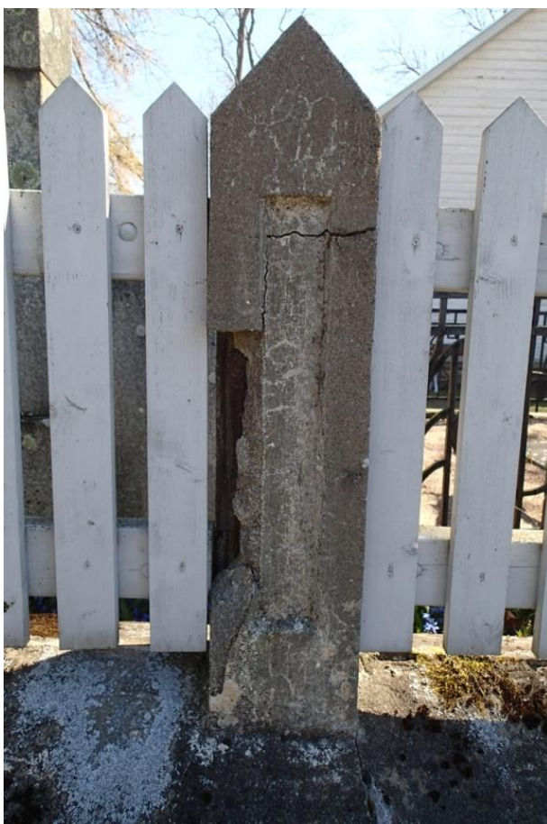
F7. Remonti vajav betoonpost
