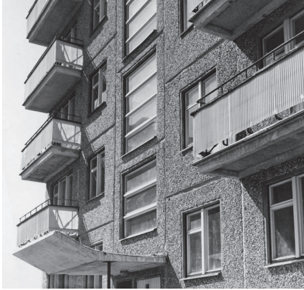
5.03: Mustamäe paneel elamu detailivaade varikatuse ja rõdudega. Detail view of prefab panel apartment buildings in Mustamäe with porch and balconies.
