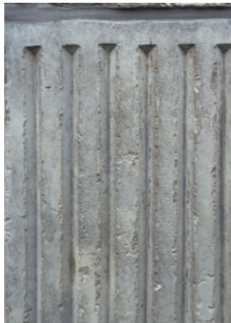
5.28: Enam-vähem korrektne reljeefse rulliga töödeldud sokli-paneel. Basement level panel with reasonably correctly stamped details.
